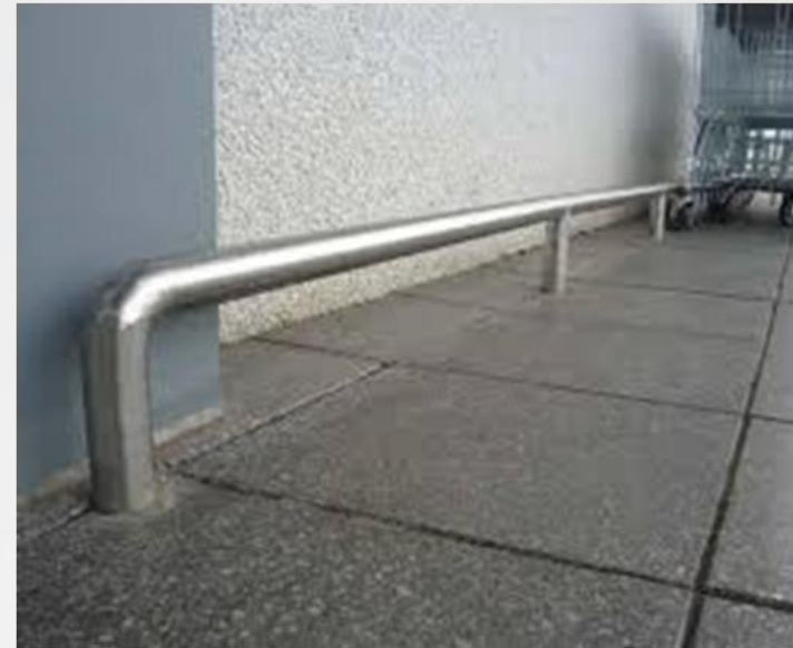
Protection against any internal vehicular or trolley movement.
