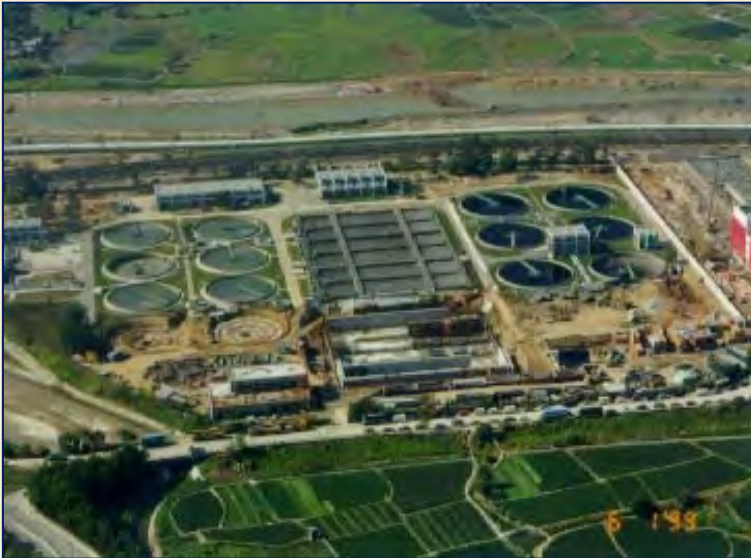
Sewage Treatment Works
